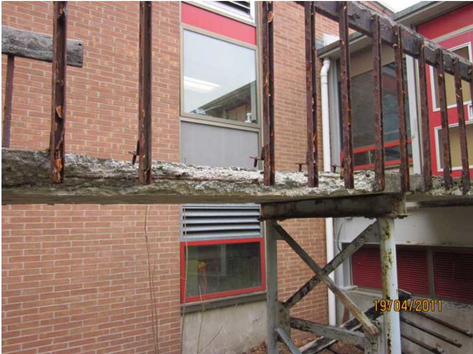
Photo 5: Corroded concrete and steel at bridge on west side of auditorium.
