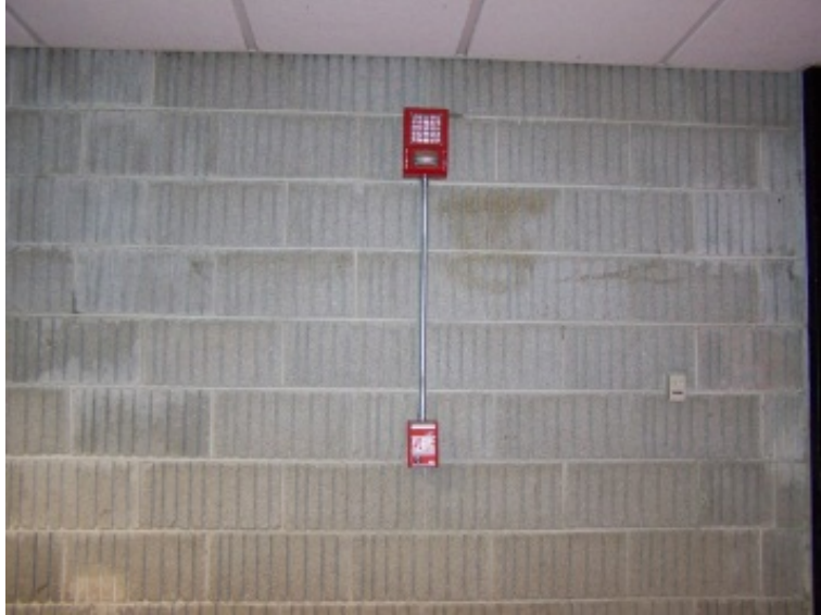
Typical Fire Alarm Components
