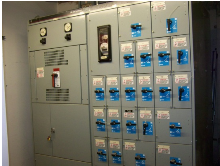
Main School switchboard
