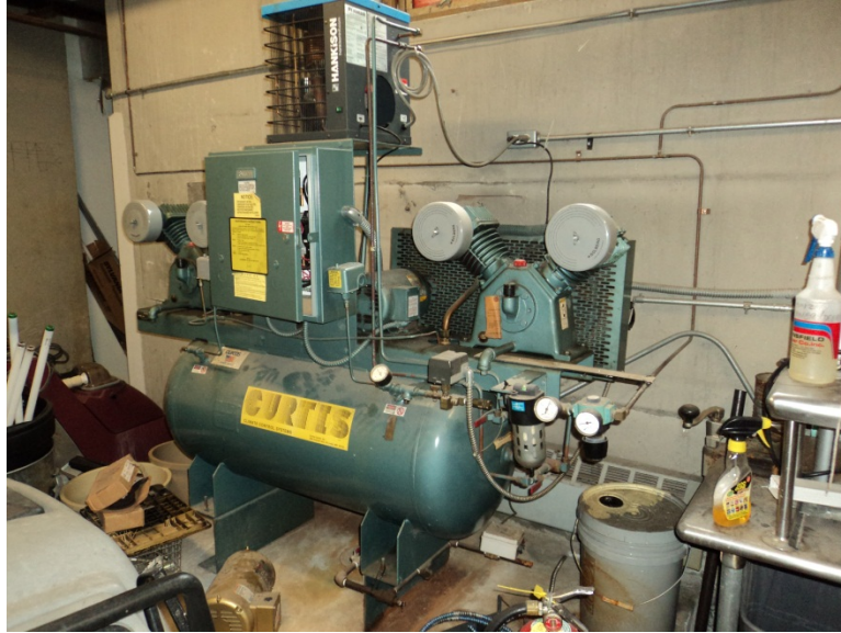
Pneumatic Controls Compressor
