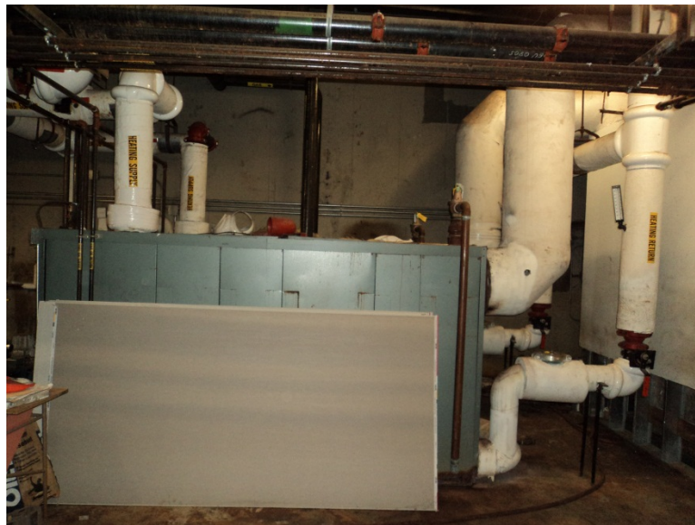
Existing Hot Water Boiler With Insulated Piping
