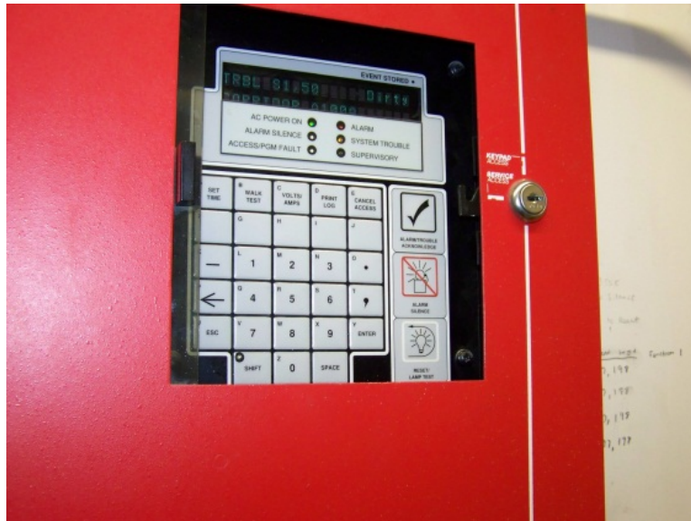
Main Fire Alarm Control Panel
