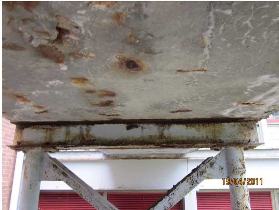
Photo 7: Corroded concrete and steel at bridge on west side of auditorium.
