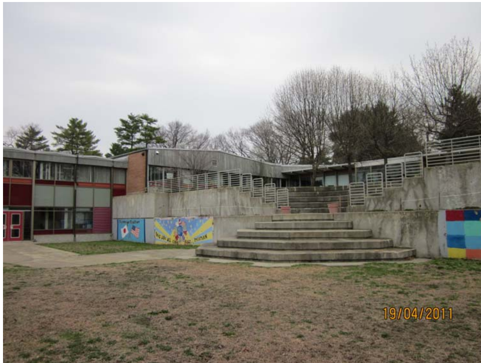
Photo 19: Condition of amphitheater concrete.
