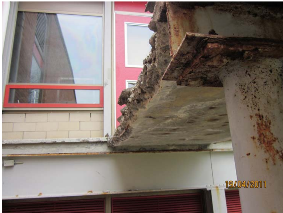
Photo 8: Corroded concrete and steel at bridge on west side of auditorium.
