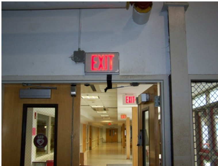
Typical Egress Lighting and Exit Signs
