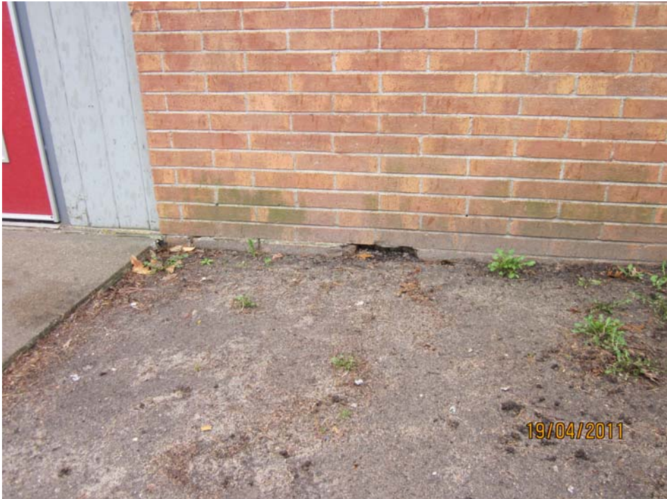
Photo 2: Brickwork cracking and decay at brick/pavement interface.
