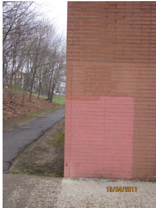
Photo 15: Brick cracking at southwest Gymnasium Two corner.
