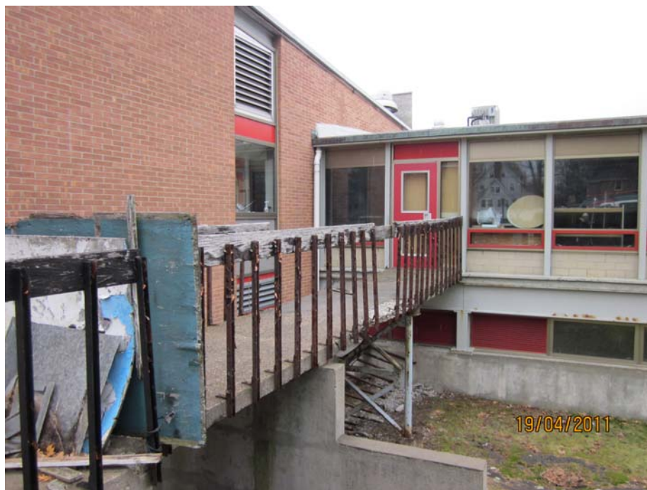
Photo 4: Corroded concrete and steel at bridge on west side of auditorium.
