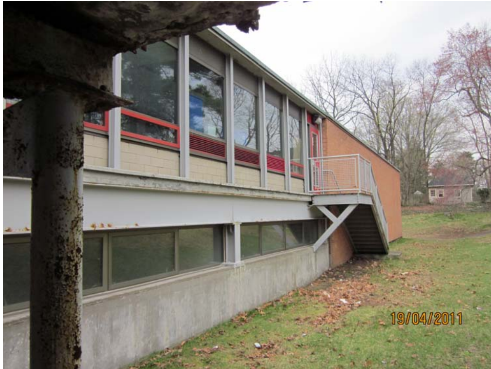
Photo 9: Corroded concrete and steel at bridge on west side of auditorium.
