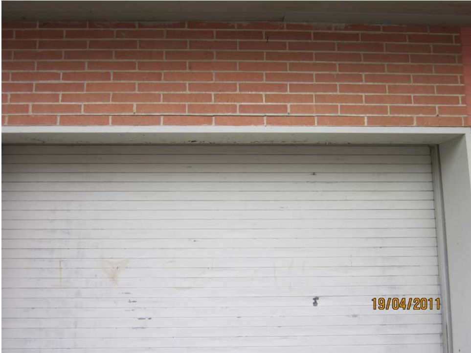
Photo 18: Brick cracking at course above overhead door in receiving.
