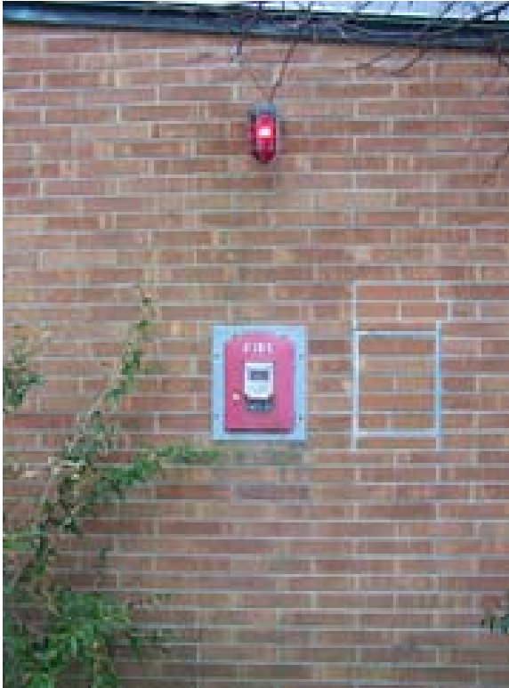
Fire Alarm Masterbox
