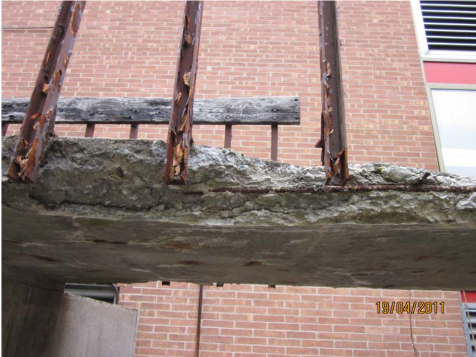
Photo 6: Corroded concrete and steel at bridge on west side of auditorium.
