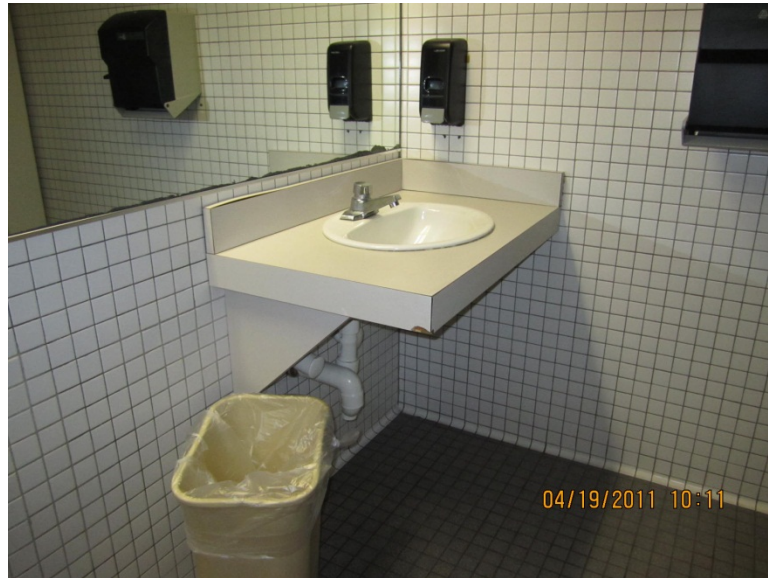
Typical Lavatory Fixture
