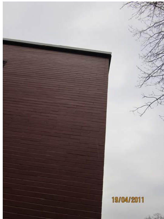
Photo 14: Localized bowing of brick at southwest Gymnasium Two corner.
