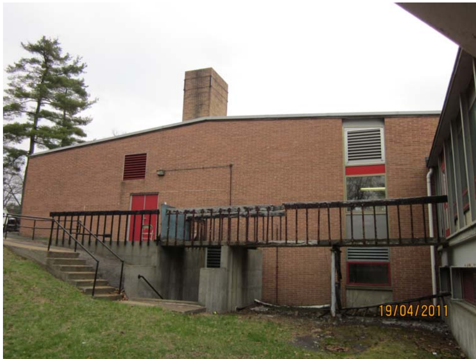
Photo 10: Corroded concrete and steel at bridge on west side of auditorium.
