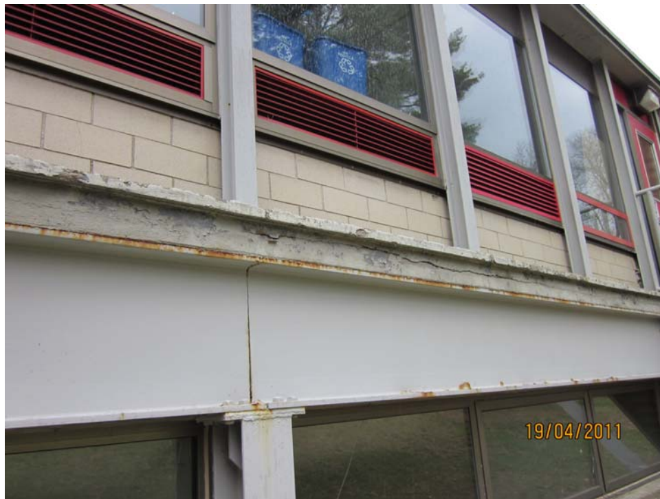
Photo 11: Slab cracking due to moisture and corrosion at exterior of band room.
