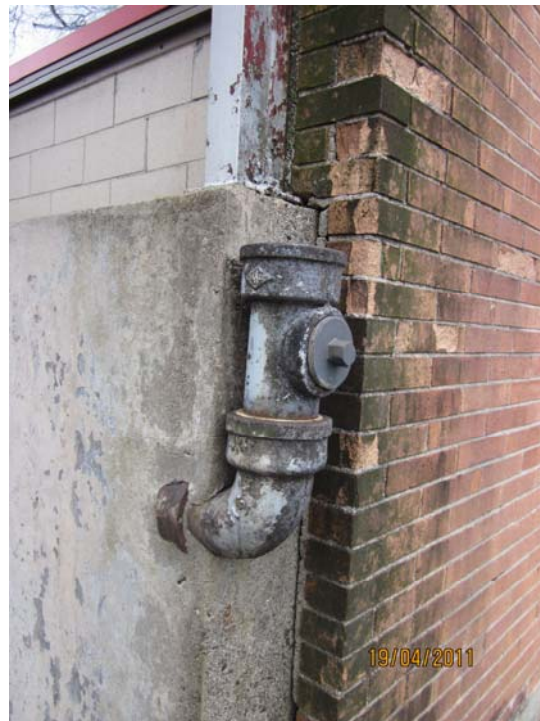
Photo 20: Brick distress at south corners of single story academic wing caused by rain leader problems.
