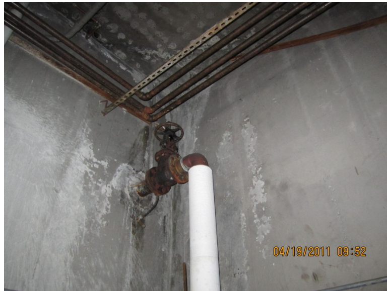
Water Service Entry
