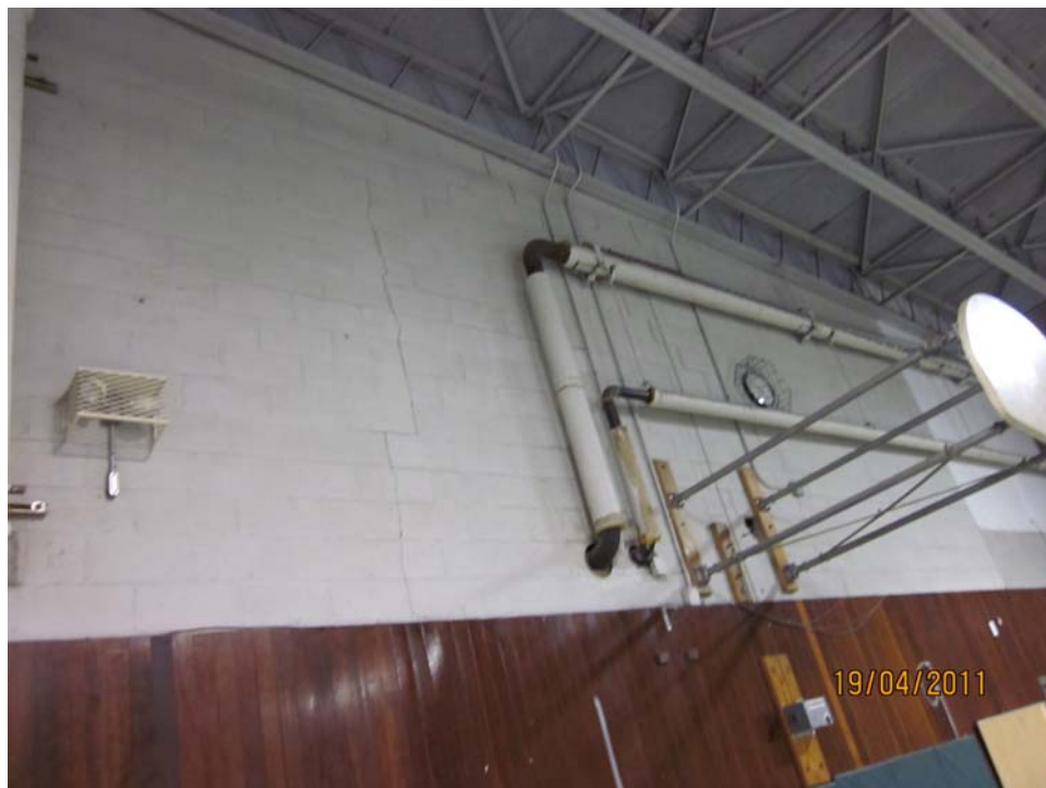
Photo 22: Interior block cracking at the gymnasium.
