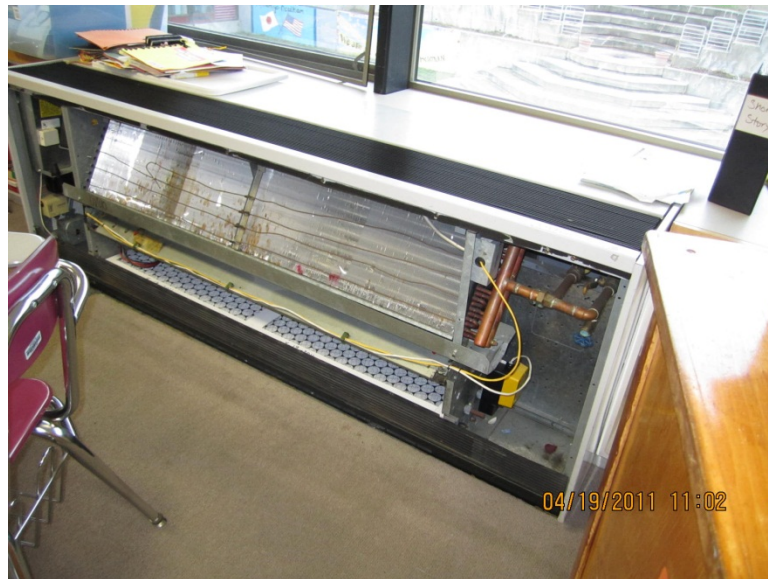
Unit Ventilator With Front Cover Removed
