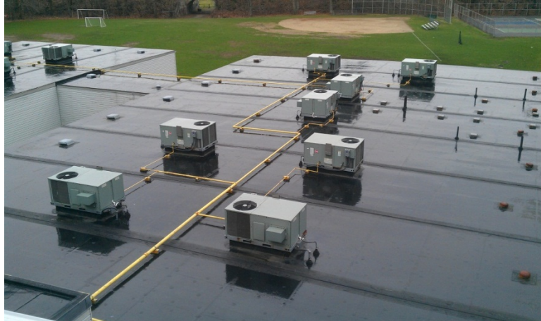
Modular Classroom Roof Showing Gas Fired Roof Top Units
