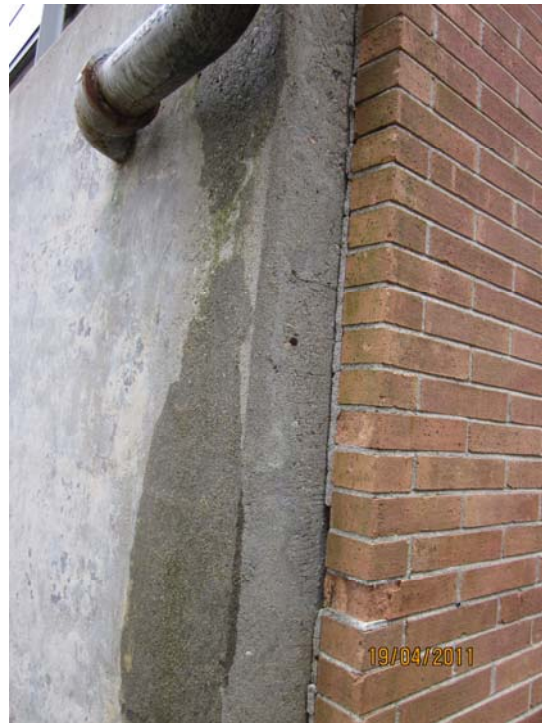
Photo 21: Brick distress at south corners of single story academic wing caused by rain leader problems.
