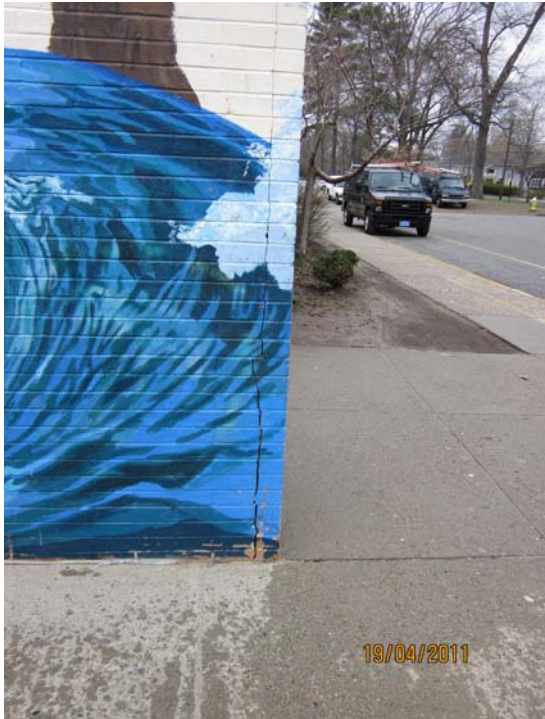
Photo 1: Brickwork cracking and decay at brick/pavement interface.
