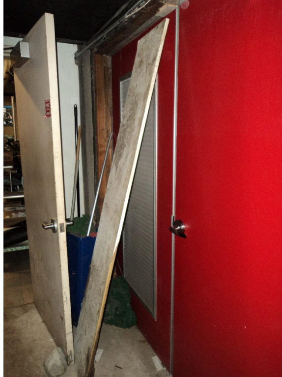
Boiler Room Combustion & Ventilation Air Intake Louver
