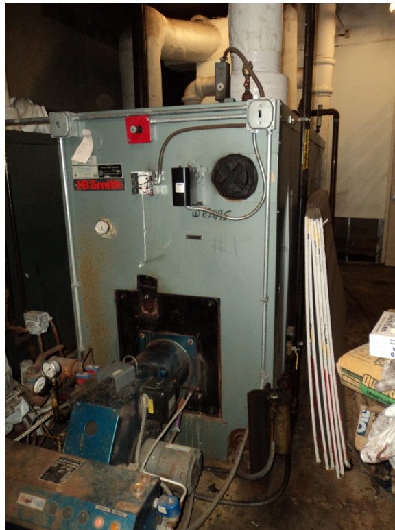
Typical Existing Hot Water Boiler
