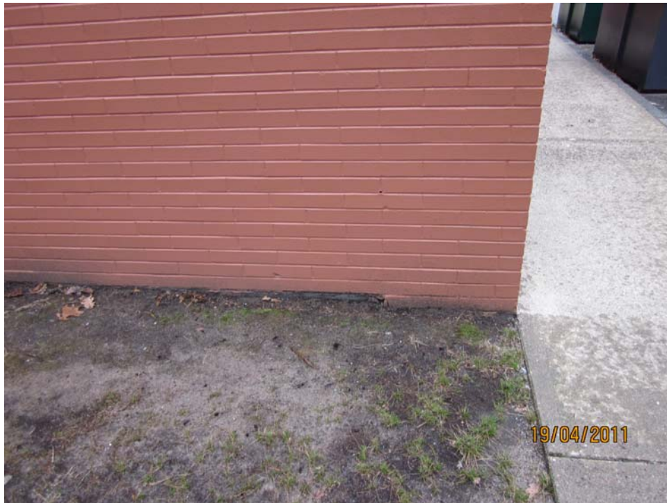
Photo 13: Decay at brick/sidewalk interface at southwest Gymnasium Two corner.
