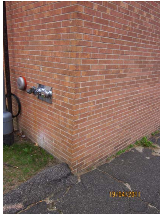
Photo 3: Brickwork cracking and decay at brick/pavement interface.
